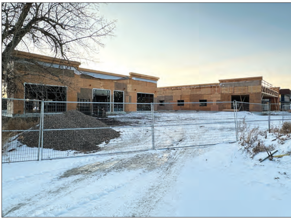
Construction continues on a day care and a seven bay commercial site continue at 1103 3rd Street West. The city's municipal planning commission approved the construction of both buildings in February 2024. | SANDRA M STANWAY PHOTO
