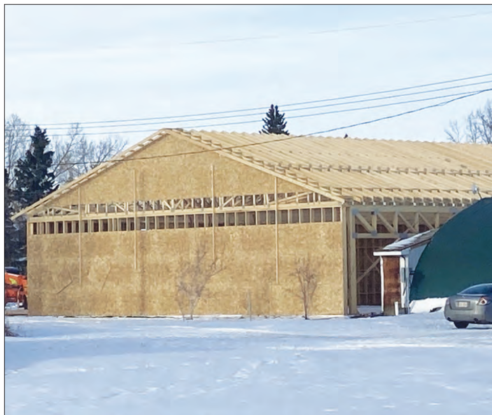
The new Scandia Hall is framed as work and fundraising continues. In September, the Quonset that was used as a hall was removed to make way for an updated structure. When the hall was taken down, some of the flooring was saved to be used as a donor recognition board in the new hall. | SUBMITTED PHOTO
