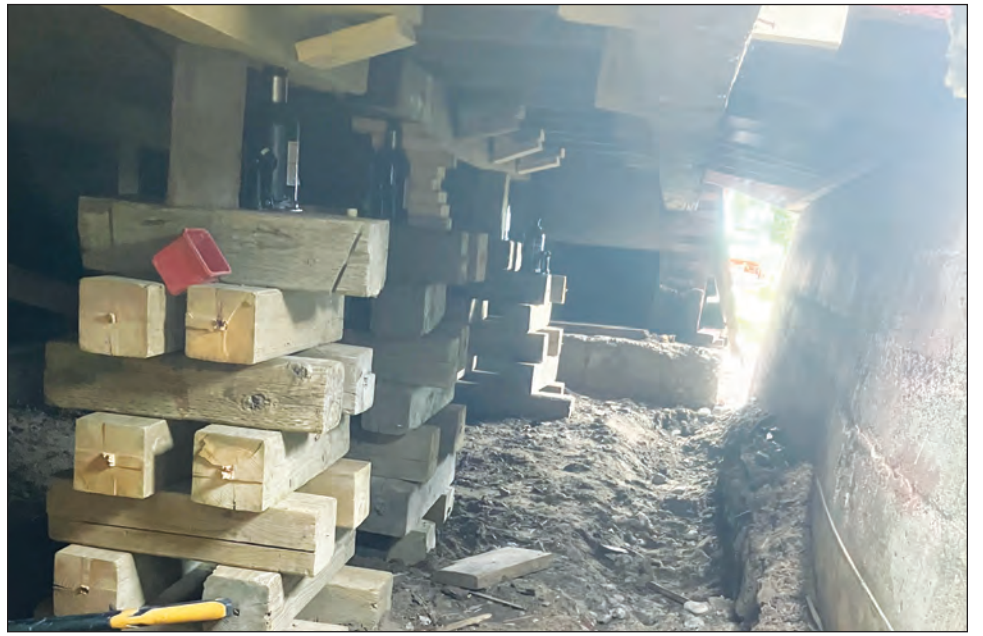
An early photo of the foundation repair under Scandia's historical elevator. Much of the work is now completed, however, other repairs need to take place but the EID Historical Park board allocated its funds into the repairs and is now seeking donations. | SUBMITTED PHOTO
