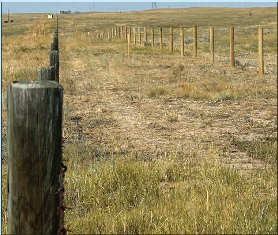
Fencing is being installed along the final 4.3km stretch of the path to Kinbrook Island Provincial Park from Township 18-2 to Bantry Bay. | SANDRA M STANWAY PHOTO
