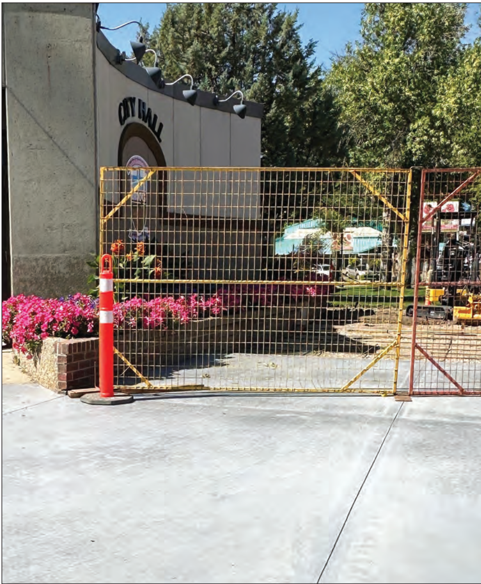
The red brick in front of city hall is being replaced with a cement walkway. The brick had been lifting and required replacement. The work was budgeted for 2024 at a cost of $80,000. | SANDRA M STANWAY PHOTO
