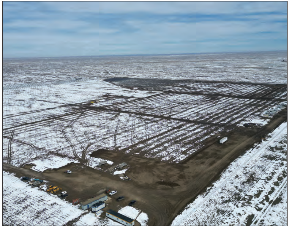
Work is underway at the Tilley Solar Project east of Tilley. As of April 2 all of the piles were installed and 18 per cent of the racking was completed. The company recently began installation of solar panels.
